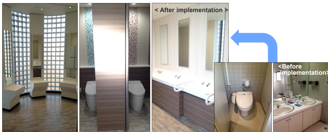
Renovation Works on Bathrooms and Kitchens on Each Floor (Tokyu Ikejiri-ohashi Building)
